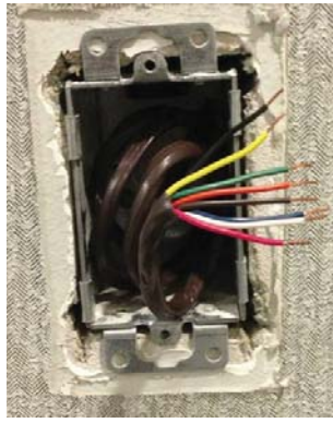
Fig. 2 - Coil Excess Wiring
